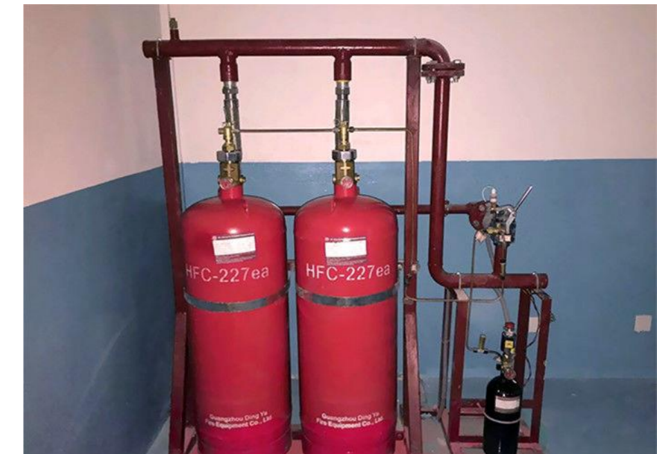
Heptafluoropropane (HFC-227ea) and perfluoro-2-methyl-3-pentanone are used in fire suppression systems.
